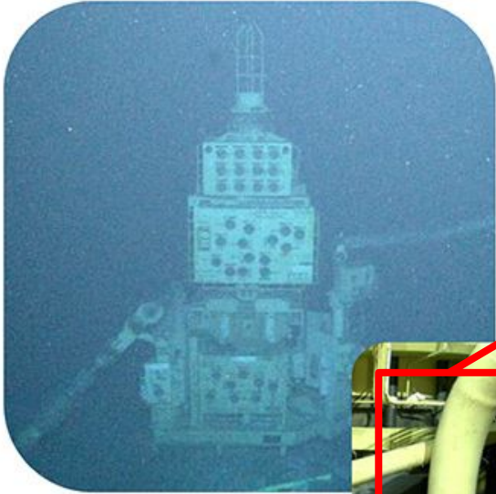
Piping of subsea equipment subject to pitting corrosion
